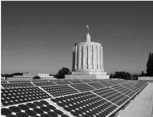
FIGURE 13.15 Solar applications on the roof of Oregon State Capital, Salem, Oregon, United States. (SMA Solar Technology AG.)
