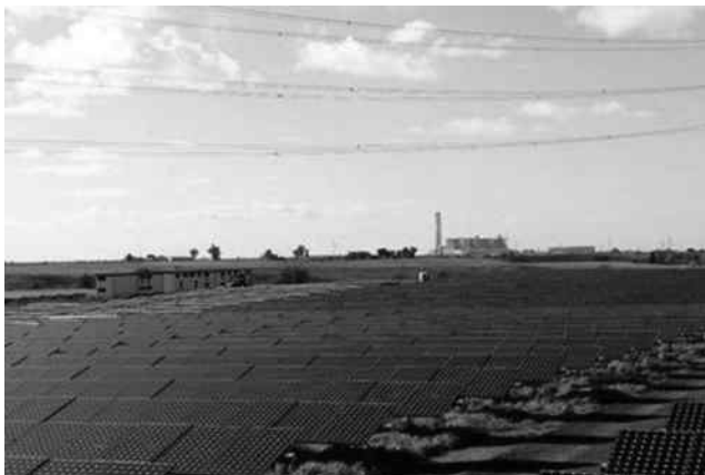
FIGURE 13.16 Solar installations at Montalto di Castro in Italy. (SMA Solar Technology AG.)
